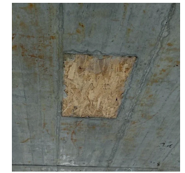
After removing the formwork, remove the OSB blind panel. The loudspeaker can then be installed.
